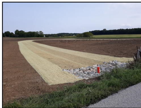
New grassy waterway & drainage rock structure on 9-17-2020 on a property in the project area.
